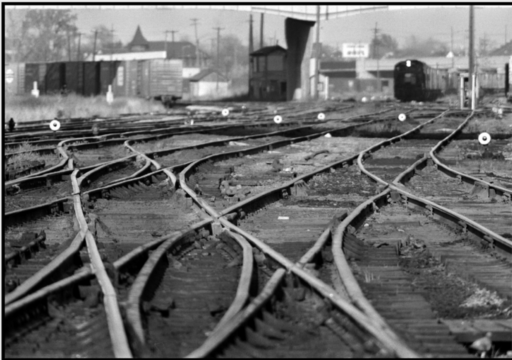
Deteriorating track work is the rule rather than the exception on the Penn Central of 1971. The 'puzzle' switches at the east end of the station platforms have seen better days. Meanwhile, a westbound mail train approaches the station and brings with it a good hour of switching.
